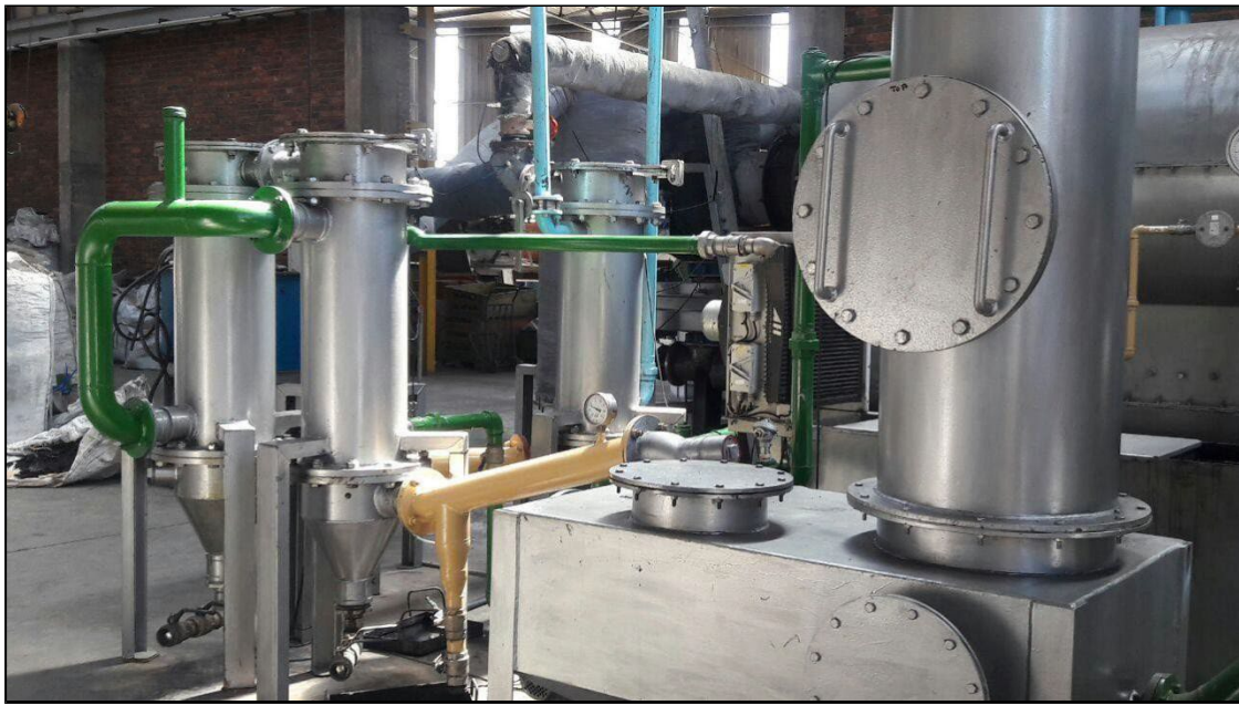
Figure 12. Photo A of a typical gas cleanup system in operation
