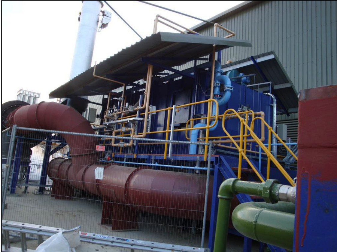
Figure 15: Photo of a typical Thermal Oxidizer in operation
