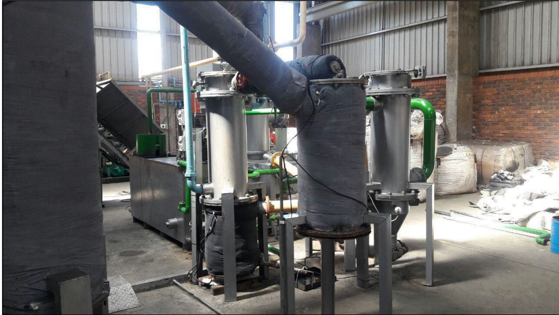
Figure 13. Photo B of a typical gas clean up system in operation
