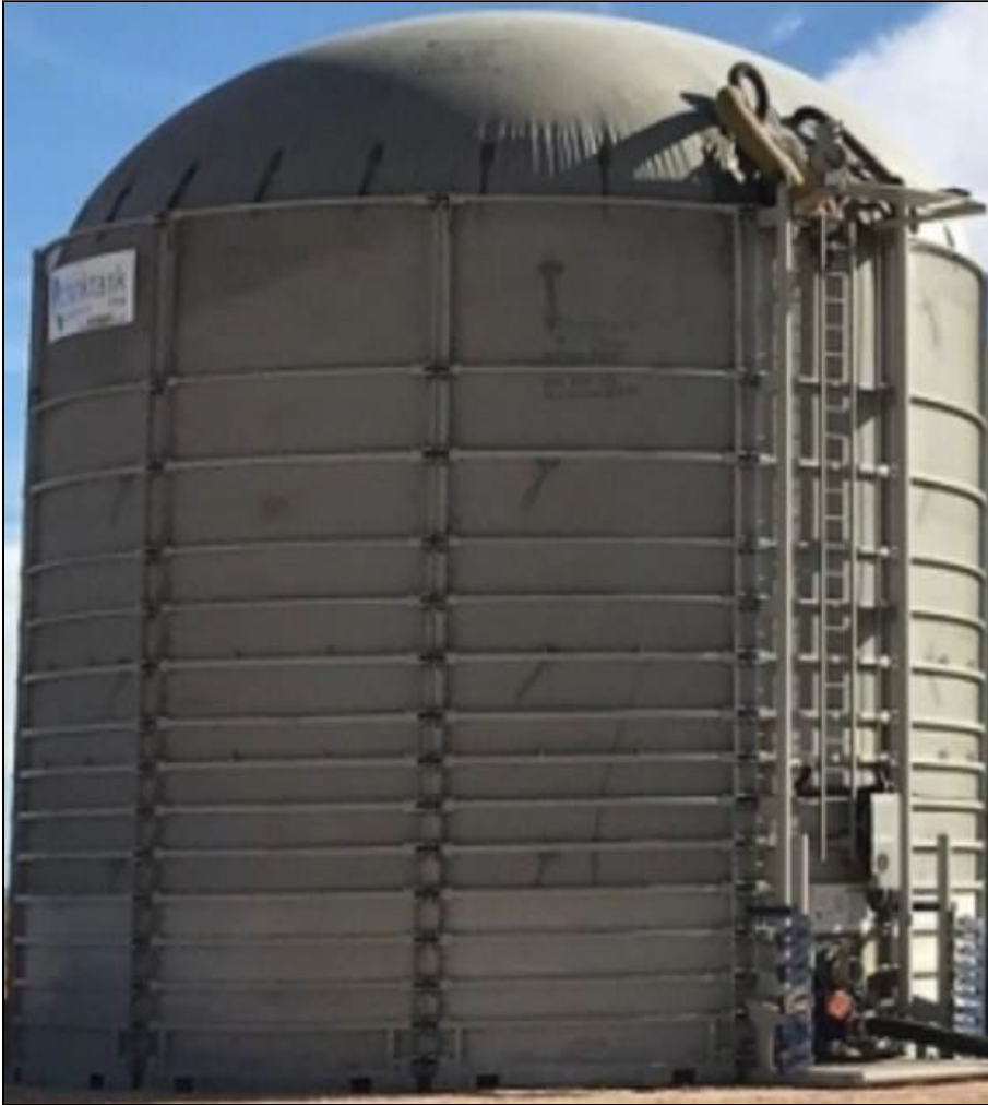
Figure 14. Picture of typical gas bladder
